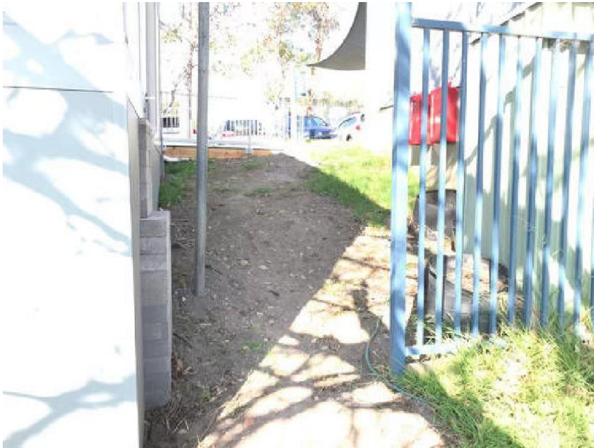
Photograph 3; Exposed soils with evidence of anthropogenic materials
